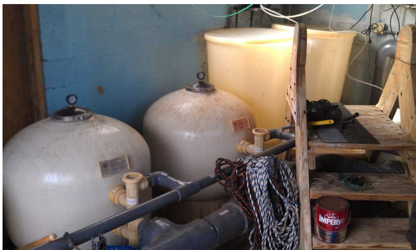
Figure 17 – Main pool filters, chemical storage, and stairs
