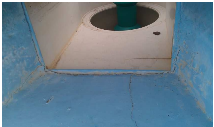
Figure 13 – Cracked joint between concrete and skimmer
