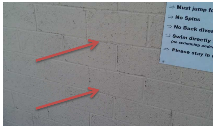
Figure 22 – Traveling cracks on filter building
