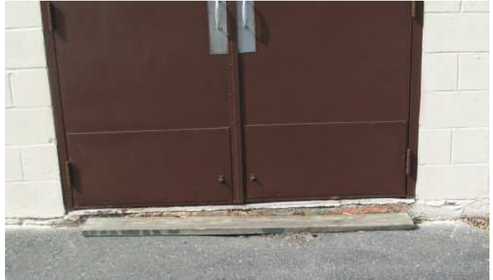
Figure 32 – Bathhouse entrance trip hazard
