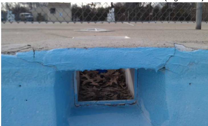
Figure 14 – Wading pool cracked coping above skimmer
